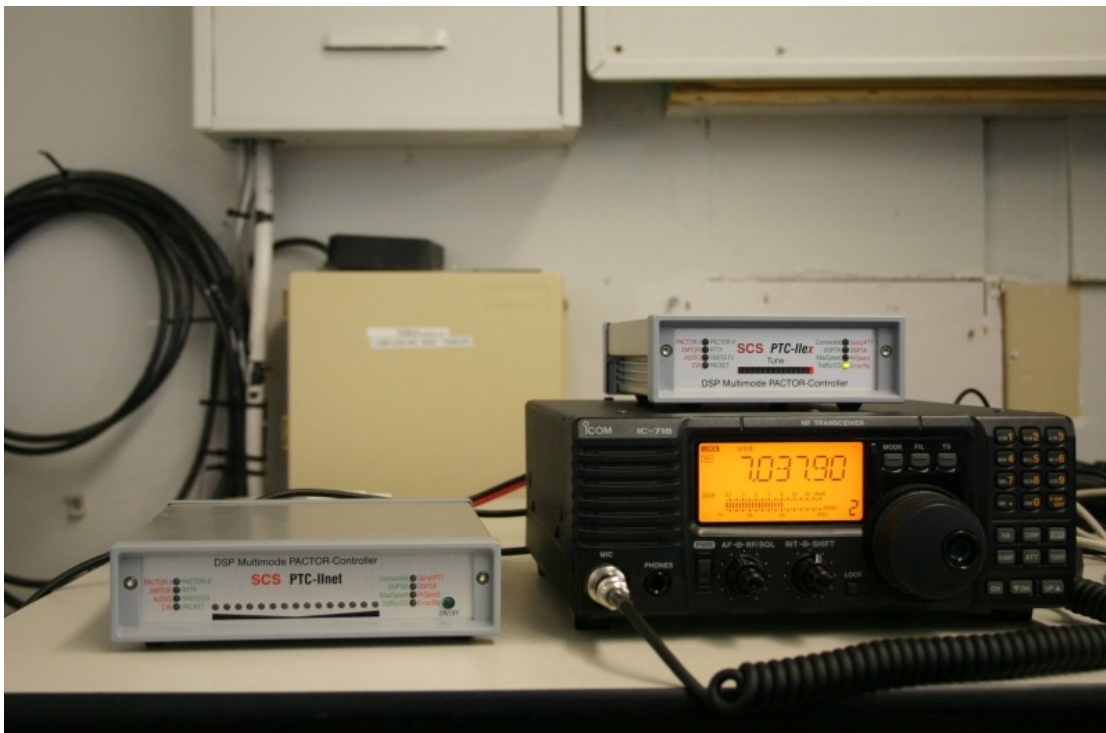
Pictured above is the equipment used in the XGATE email system. As configured the HF radio, SCS PTC-IIex and SCS PTC-IInet provides a radio to internet email gateway.
